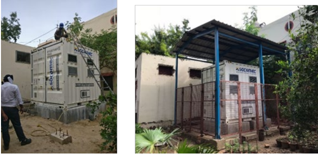
Fig. 11. Shed for the BESS
