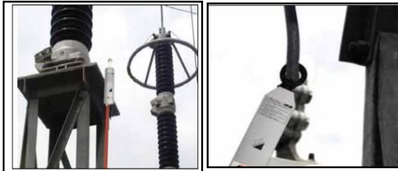
Fig. 8 CT and voltage sensing device testing positions.
