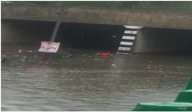
Figure 10: Water logging in underpass due to non-functional motors
