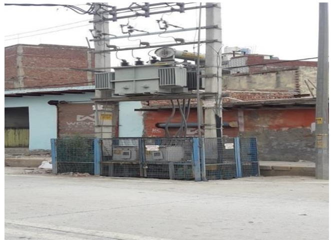
Figure 4: Dangerous electrical substation due to CC Road work in DSIDC area
