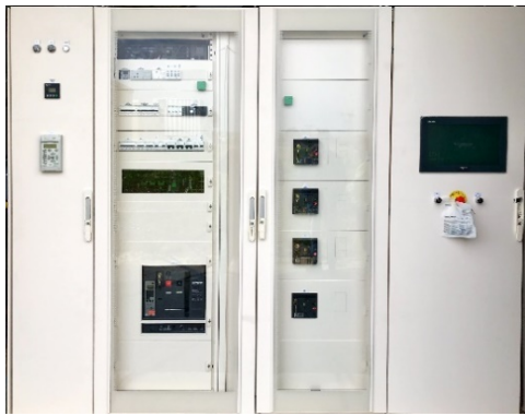
Fig. 6. View of the LV ECC switchboard
