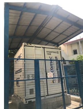
Fig. 5. View of the BESS container deployed at site.
