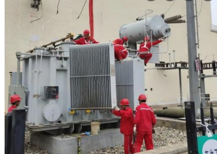
Image 10- Routine maintenance of Power Transformer
