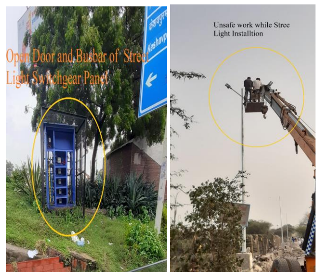
Figure 9: Unsafe Street Light Boxes and Unsafe Street Light Installation Work during road widening work
