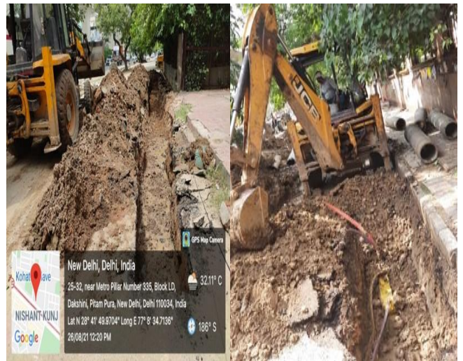
Figure 5: UG Cable damage by PWD Works
