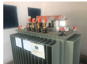
Fig. 4. View of the 630 kVA transformer at site.
