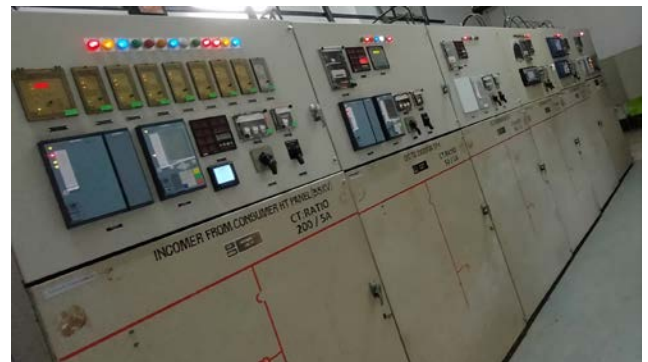
Fig. 2. L&T's Digital Substation
