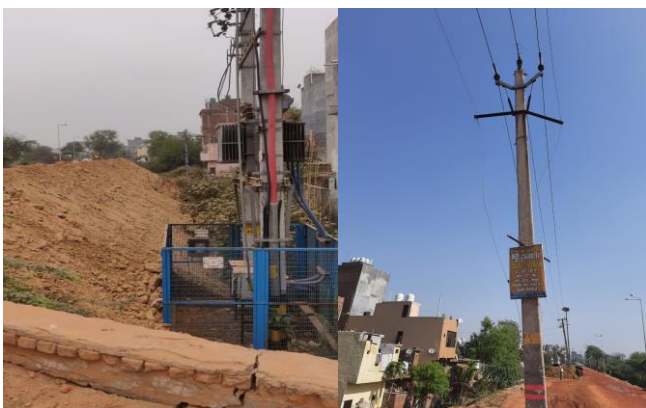
Figure 3: I&FC Road Widening work and perilous electrical network
